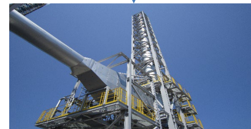
New incinerator in Yokohama
