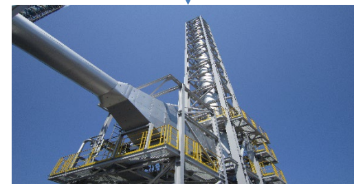
New incinerator in Yokohama
