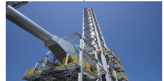
New incinerator in Yokohama
