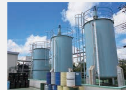
Waste oil recycling facility, Yokohama Plant, Japan Waste
